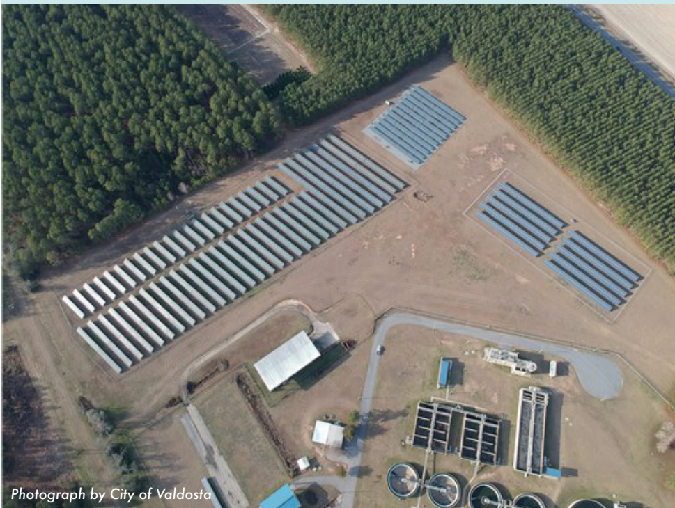
Solar installation at a Valdosta wastewater treatment plant.
