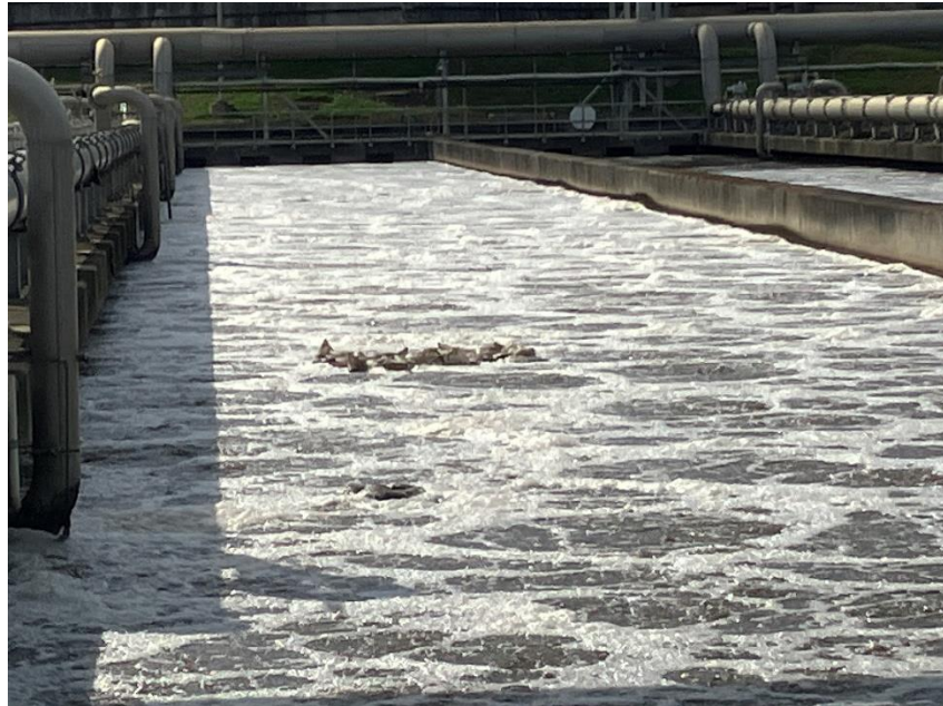
BNR Photo 4: Solids in a BNR Basin
