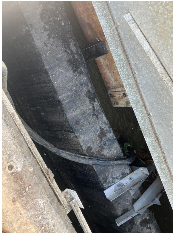
Primary Clarification Photo 2: Primary Clarifier being Mixed
