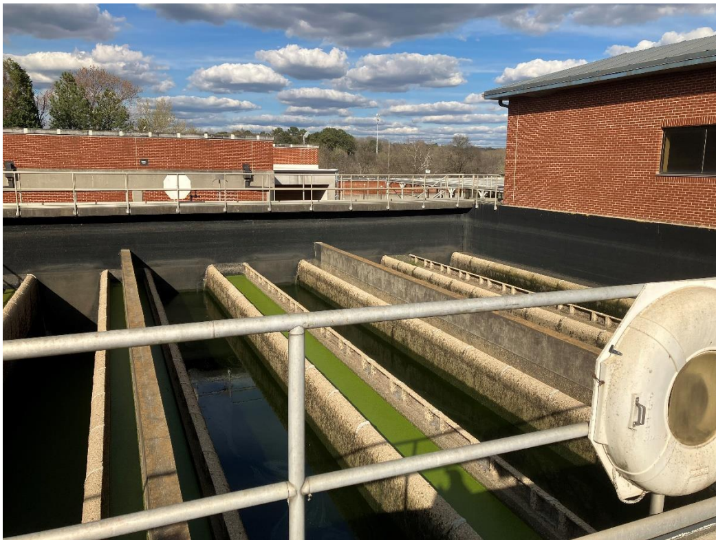
Tertiary Treatment Photo 8: Offline Sand Filters (2)
