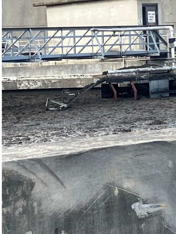
SC Photo 4: Broken arm on secondary clarifier #3
