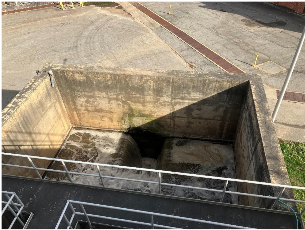
Tertiary Treatment Photo 6: Sand Filter Backwash Flow to BNRs
