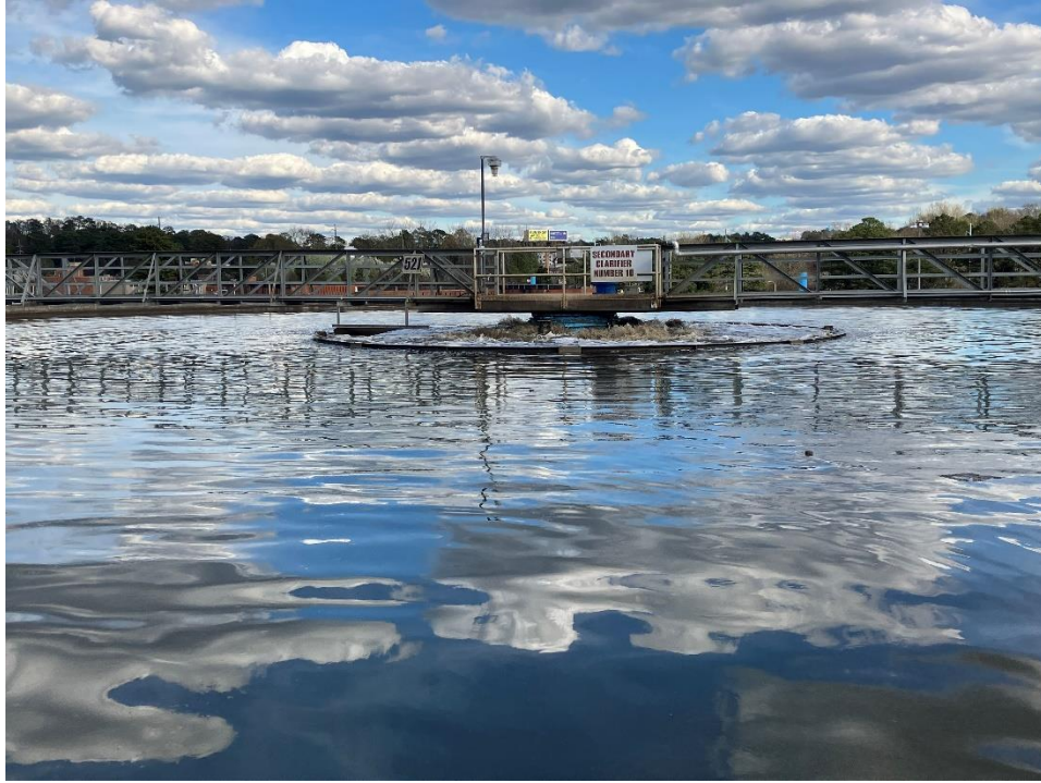
SC Photo 10: Secondary Clarifier #10
