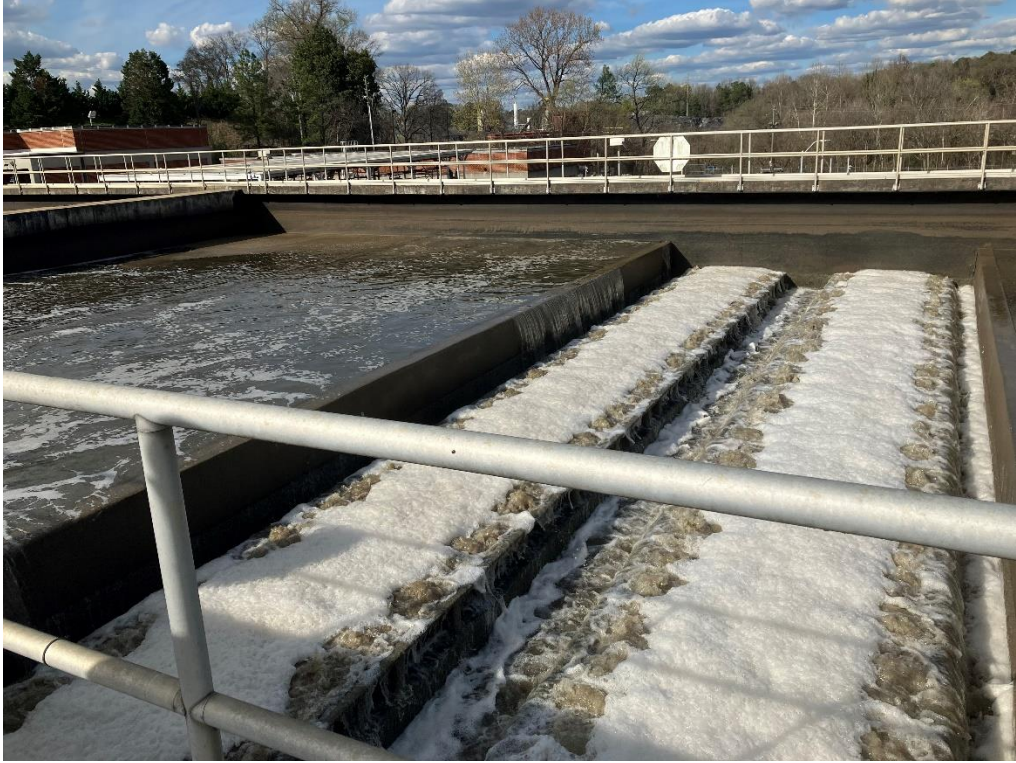
Tertiary Treatment Photo 5: Sand Filters Backwashing
