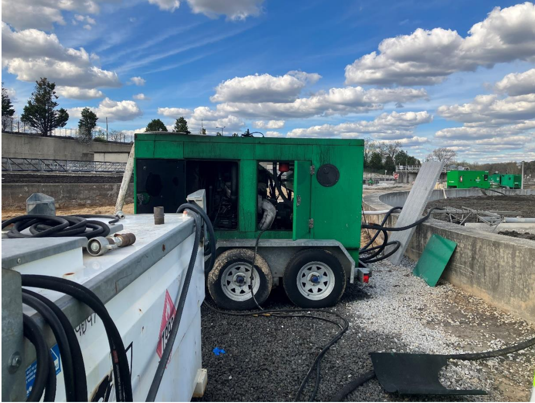
SC Photo 12: Pumps Used to Return Clarifier Flow to System
