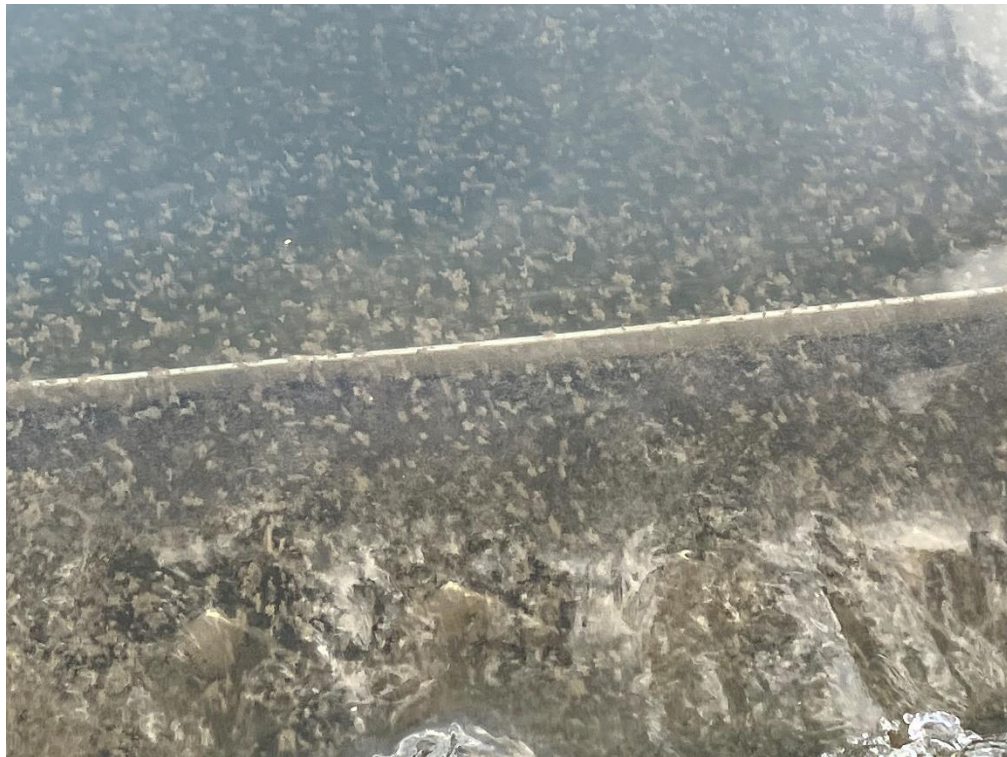
SC Photo 11: Solids in Secondary Clarifier #10 Effluent
