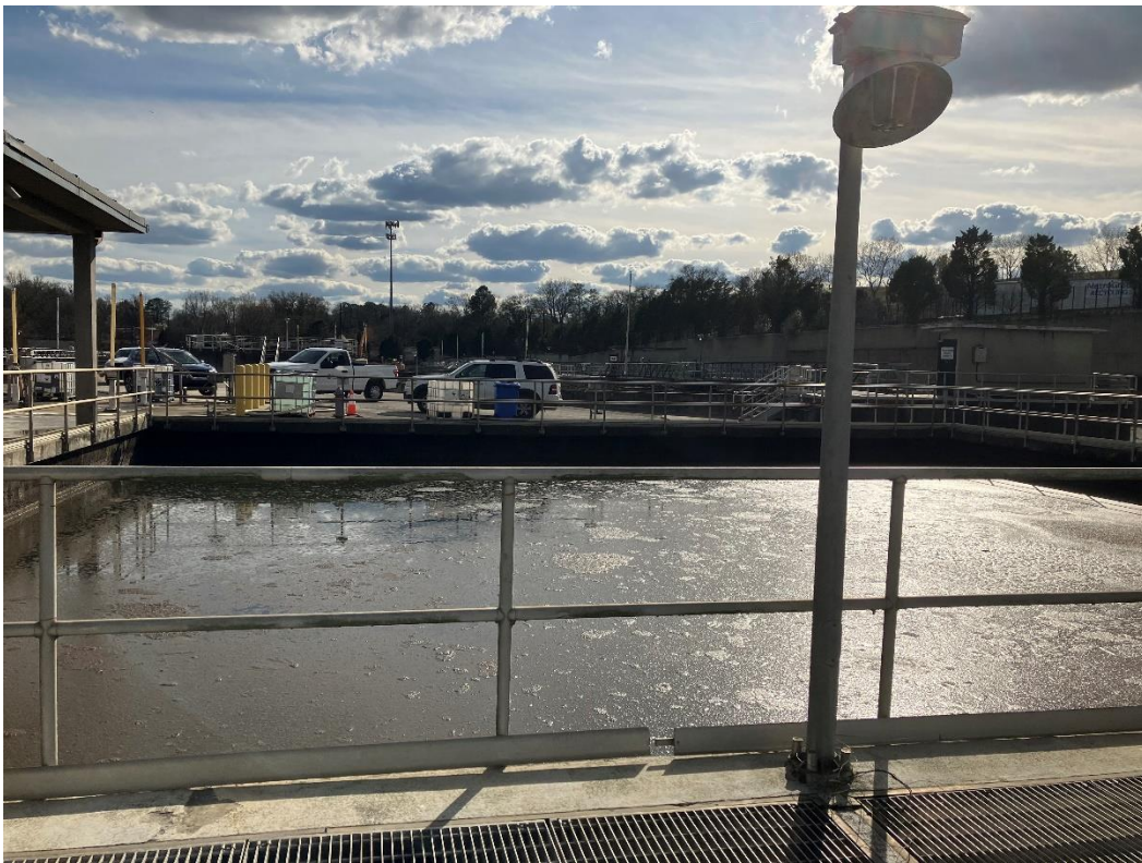
Tertiary Treatment Photo 4: Sand Filters (4)
