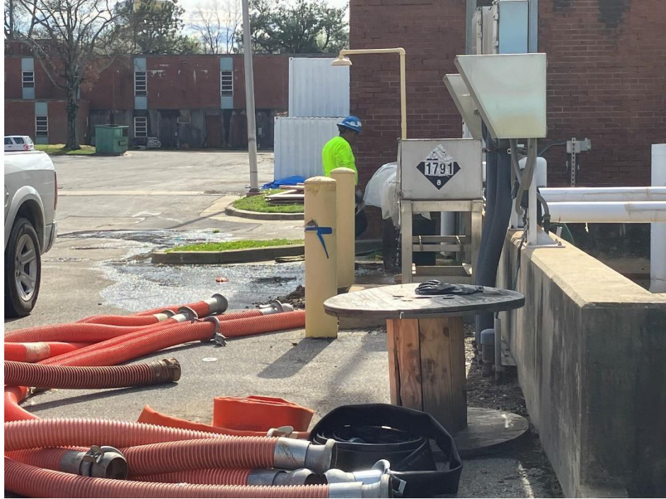
O&M Photo 3: Broken Eyewash Station (2)
