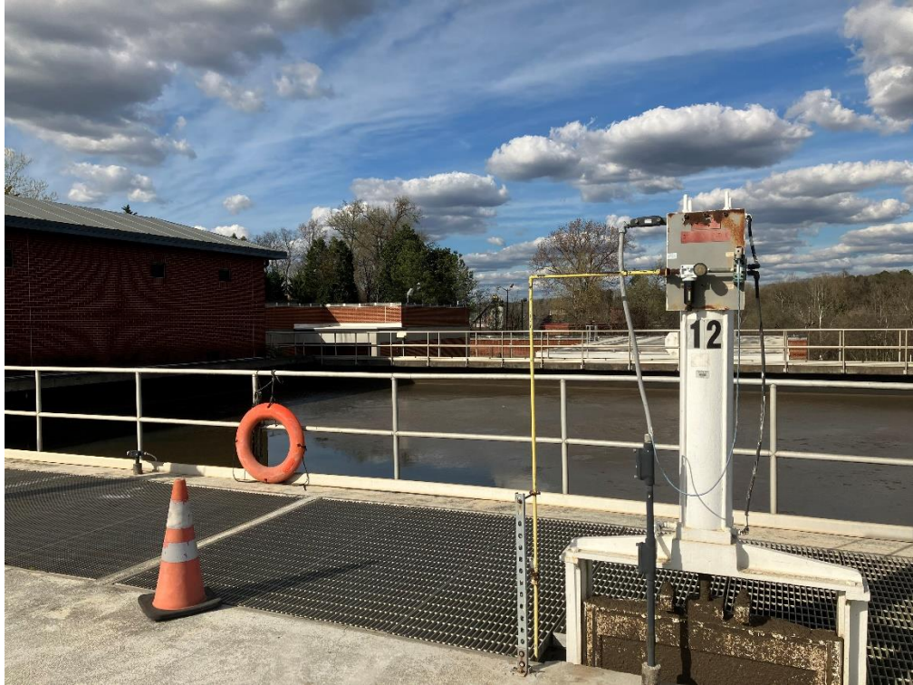
Tertiary Treatment Photo 3: Sand Filters (3)
