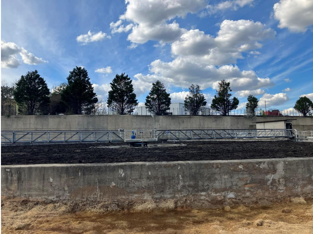
SC Photo 6: Secondary Clarifier #5
