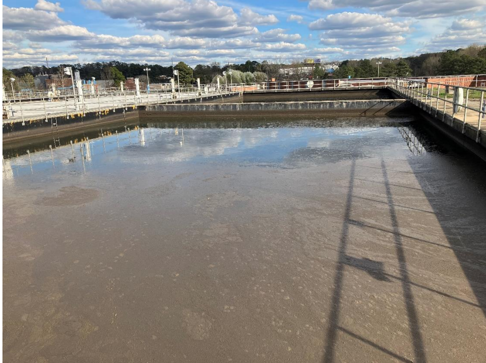
Tertiary Treatment Photo 1: Sand Filters (1)
