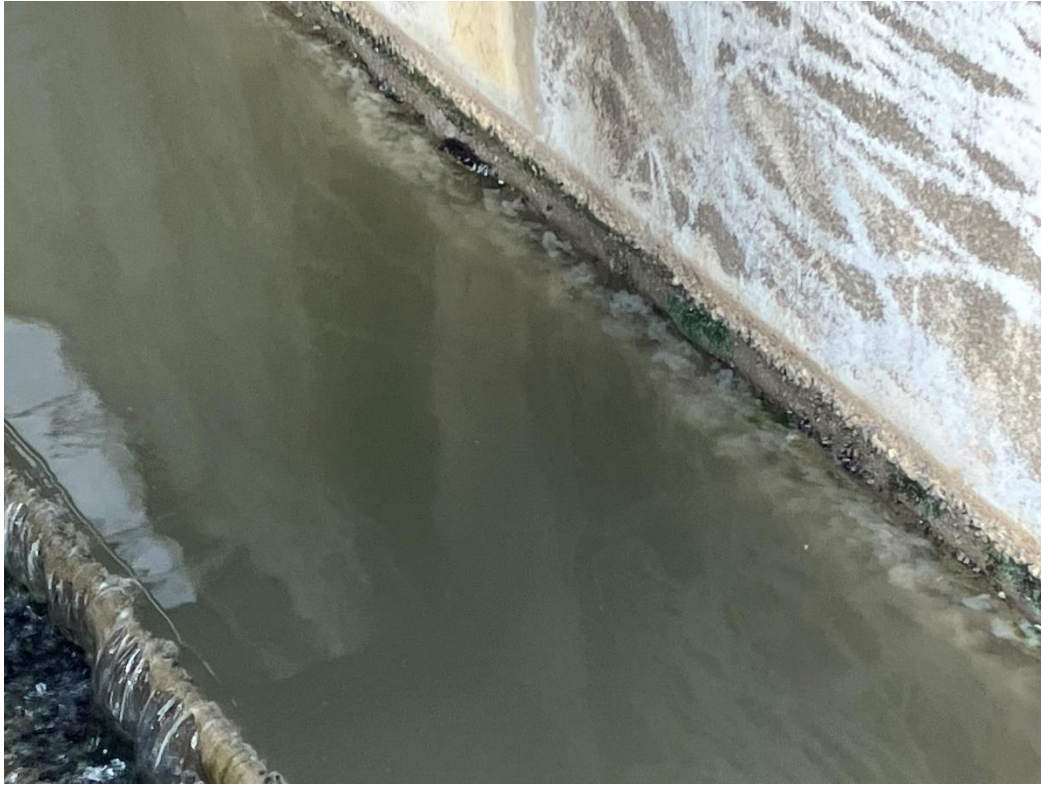
Disinfection Photo 4: Solids on Walls of UV Treated Effluent (3)
