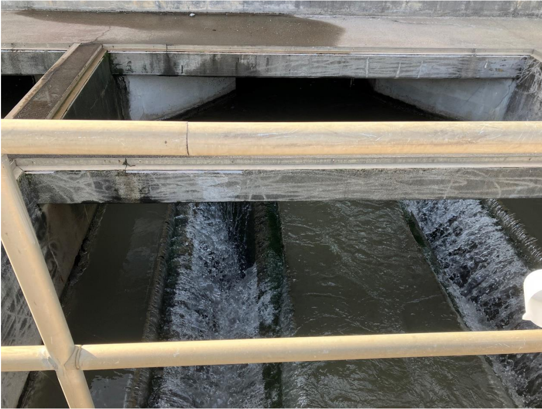
Disinfection Photo 1: UV Flow
