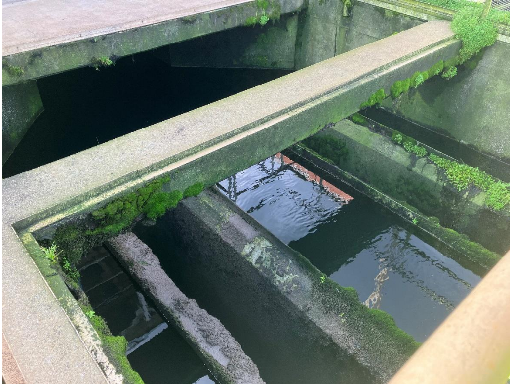
Disinfection Photo 5: Offline UV Channel
