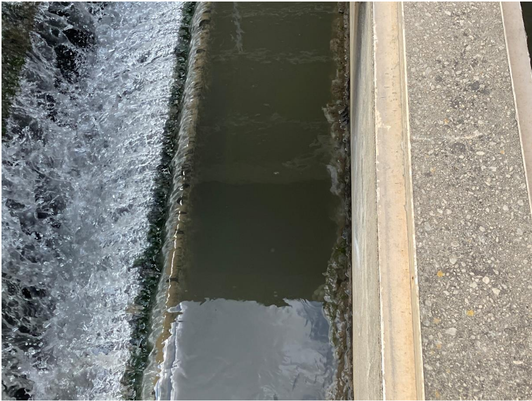
Disinfection Photo 3: Solids on Walls of UV Treated Effluent (2)
