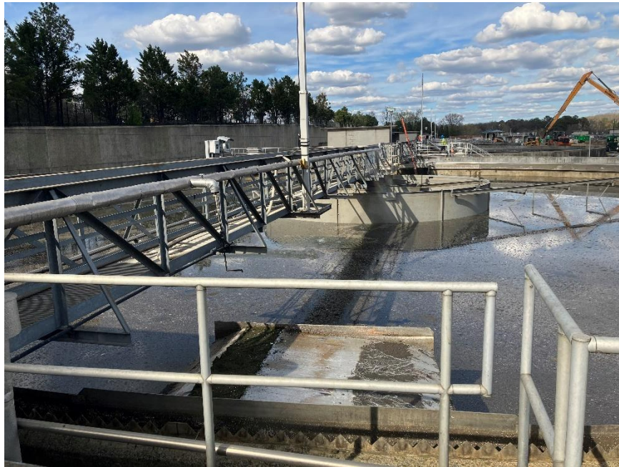
SC Photo 1: Secondary Clarifier #1
