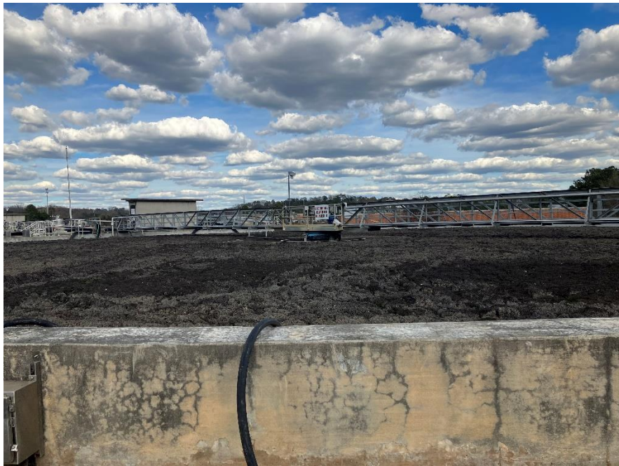
SC Photo 5: Secondary Clarifier #6
