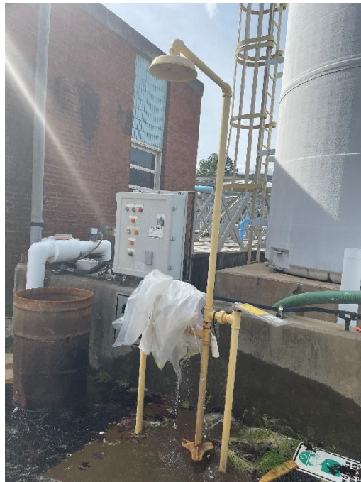
O&M Photo 2: Broken Eyewash Station (1)
