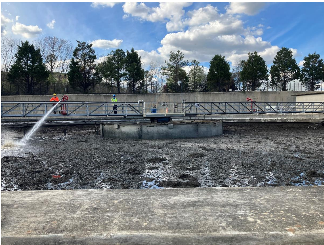
SC Photo 3: Secondary Clarifier #3
