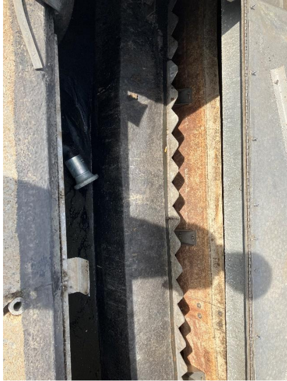
Primary Clarification Photo 1: Primary Clarifier
