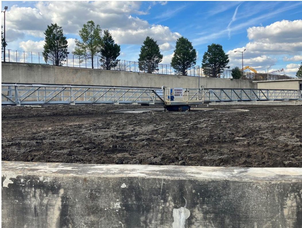
SC Photo 9: Secondary Clarifier #9
