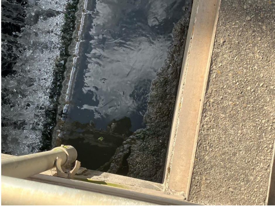
Disinfection Photo 2: Solids on Walls of UV Treated Effluent (1)
