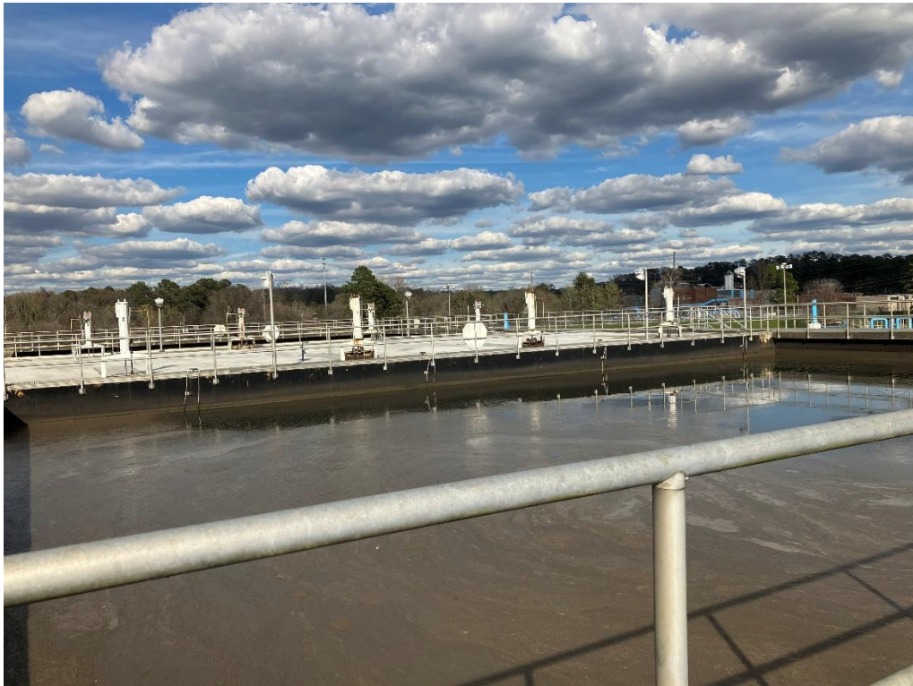
Tertiary Treatment Photo 2: Sand Filters (2)
