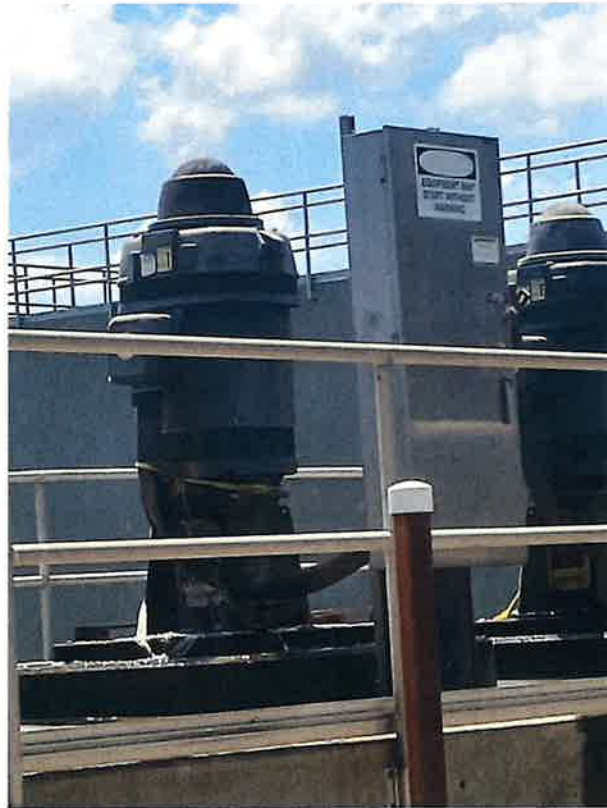
Photo 36: Damaged Equipment Near UV
