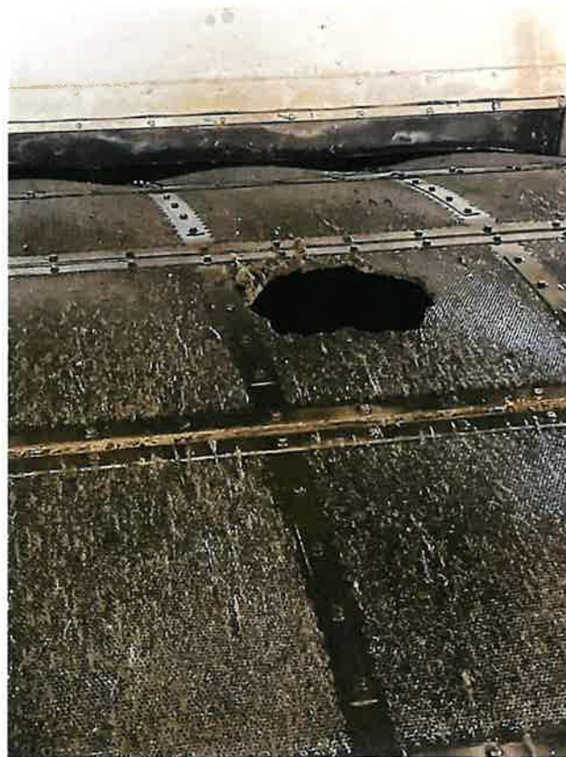
Photo 10: Damage to Drum Screen #2
