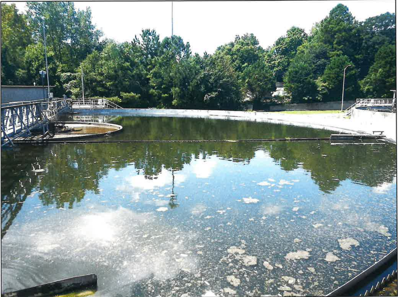
Photo 13. Secondary Clarification – Clarifier #2 with abundant floating solids and bent skimming equipment.
