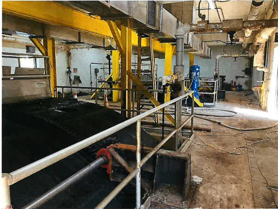
Photo 9: Drum Screens #2 and #3
