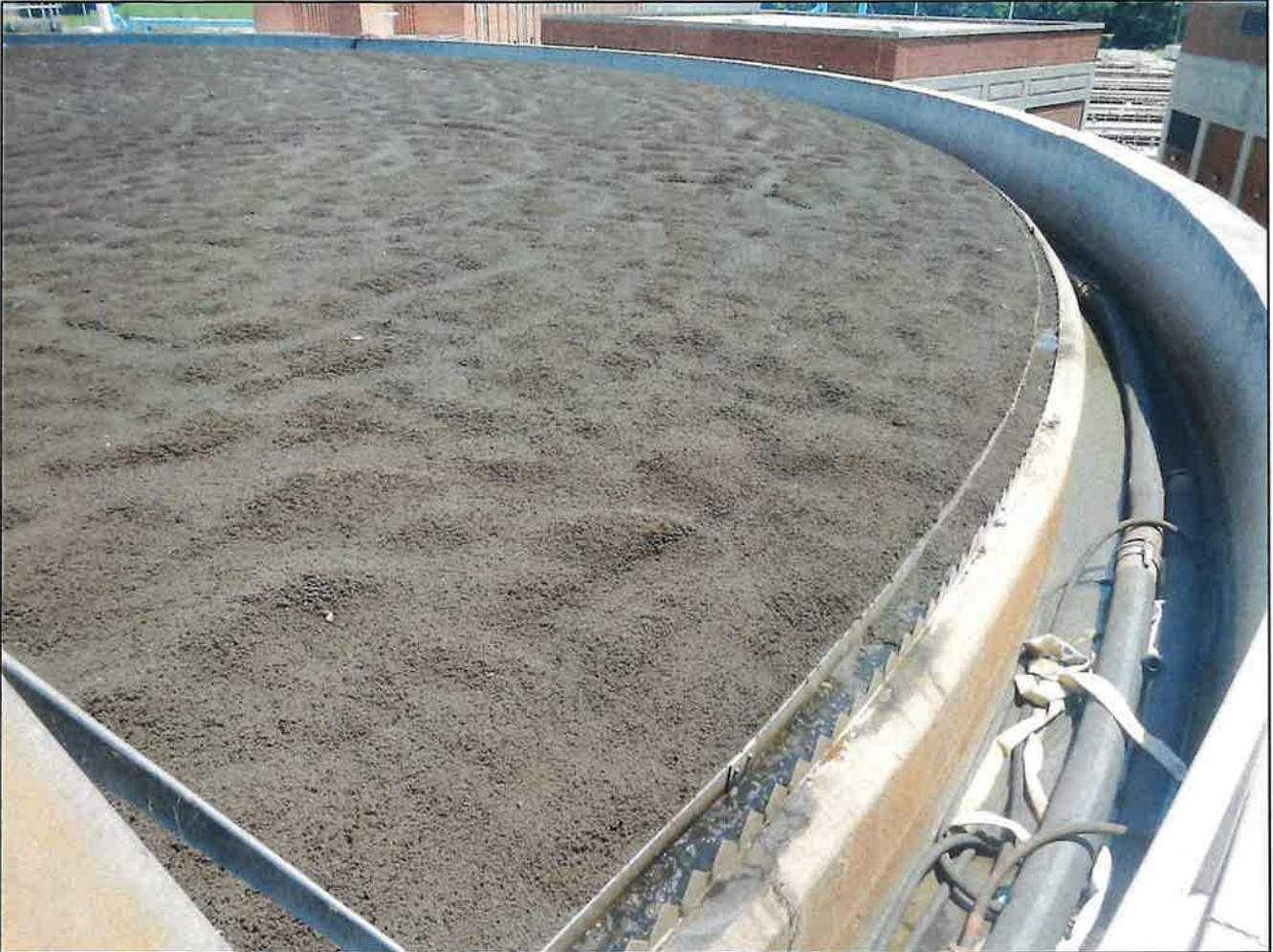
Photo 15. Secondary Clarification – Clarifier #8 (out of service) with effluent channel cleaned out and with floating solids blanket.
