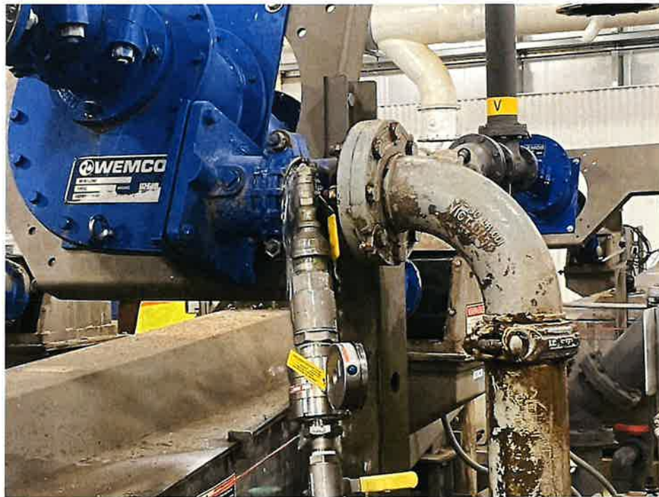
Photo 6: Damaged Grit Classifier Zoomed In
