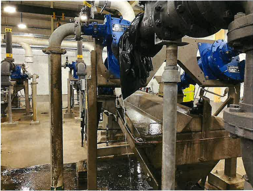
Photo 7: Damaged Grit Classifier (2)
