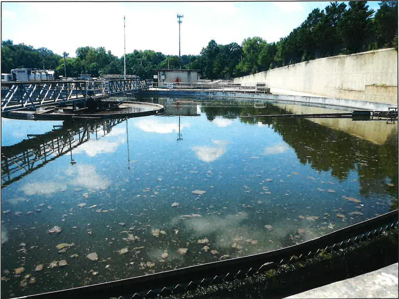
Photo 11. Secondary Clarification – Clarifier #7 with abundant floating solids and broken skimming arm.
