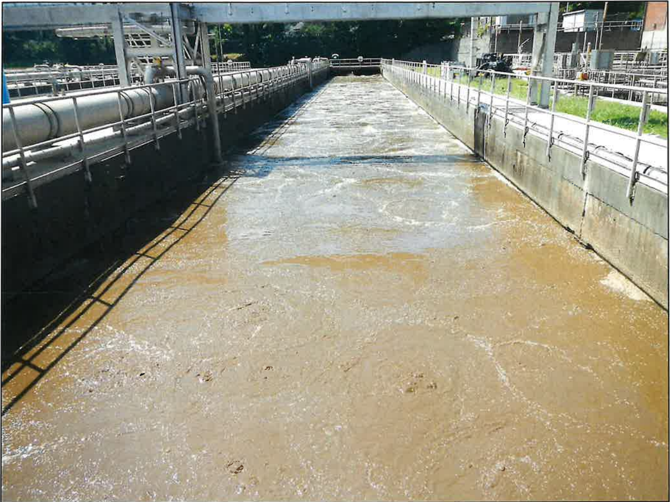
Photo 7. Biological Nutrient Removal (“BNR”) – Evidence of diffuser issues in Tank #1.
