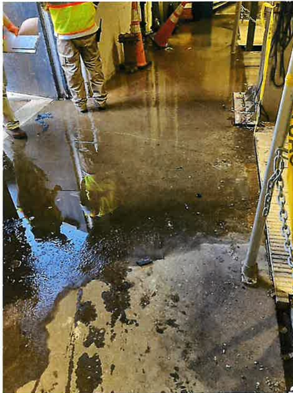
Photo 2: Leak in Bar Screen Room
