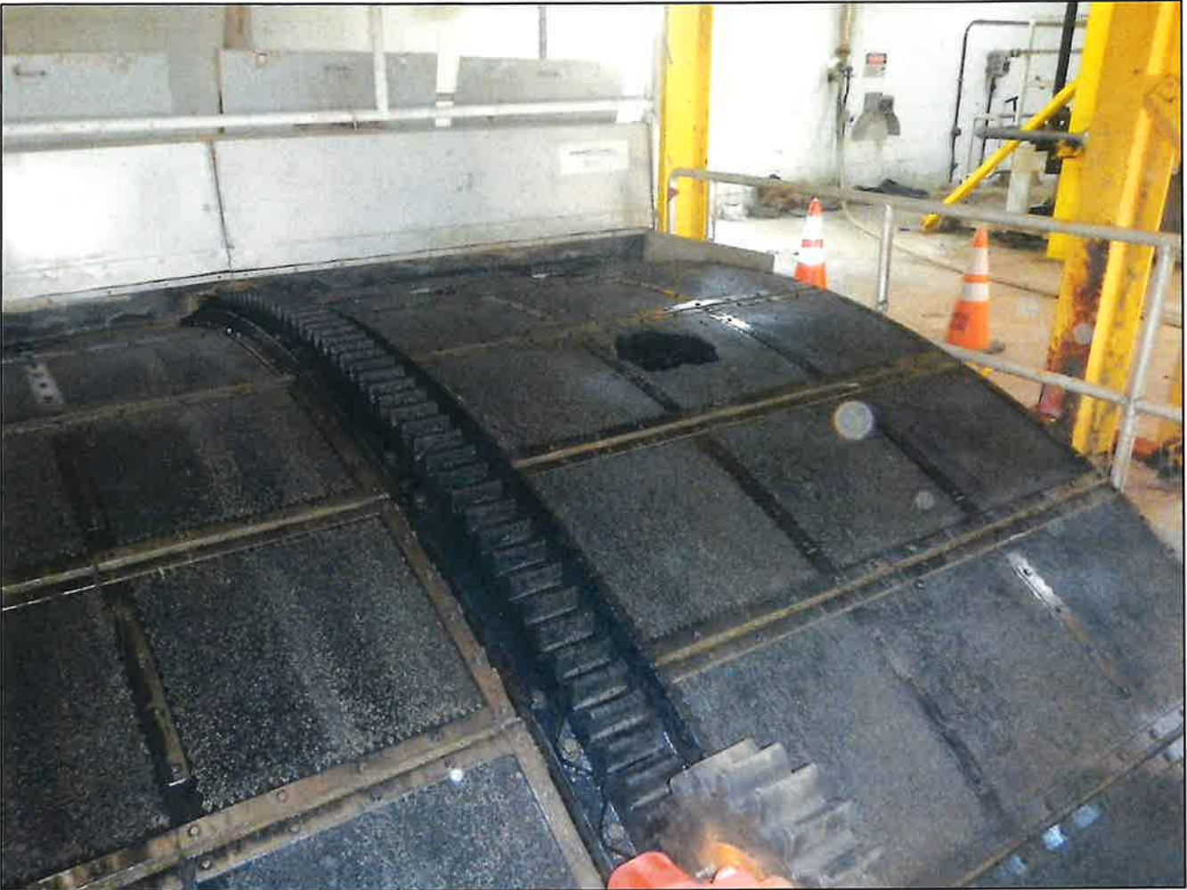
Photo 2. Primary Screening – Hole within fine mesh screen drum #2 in Drum Screen Building.
