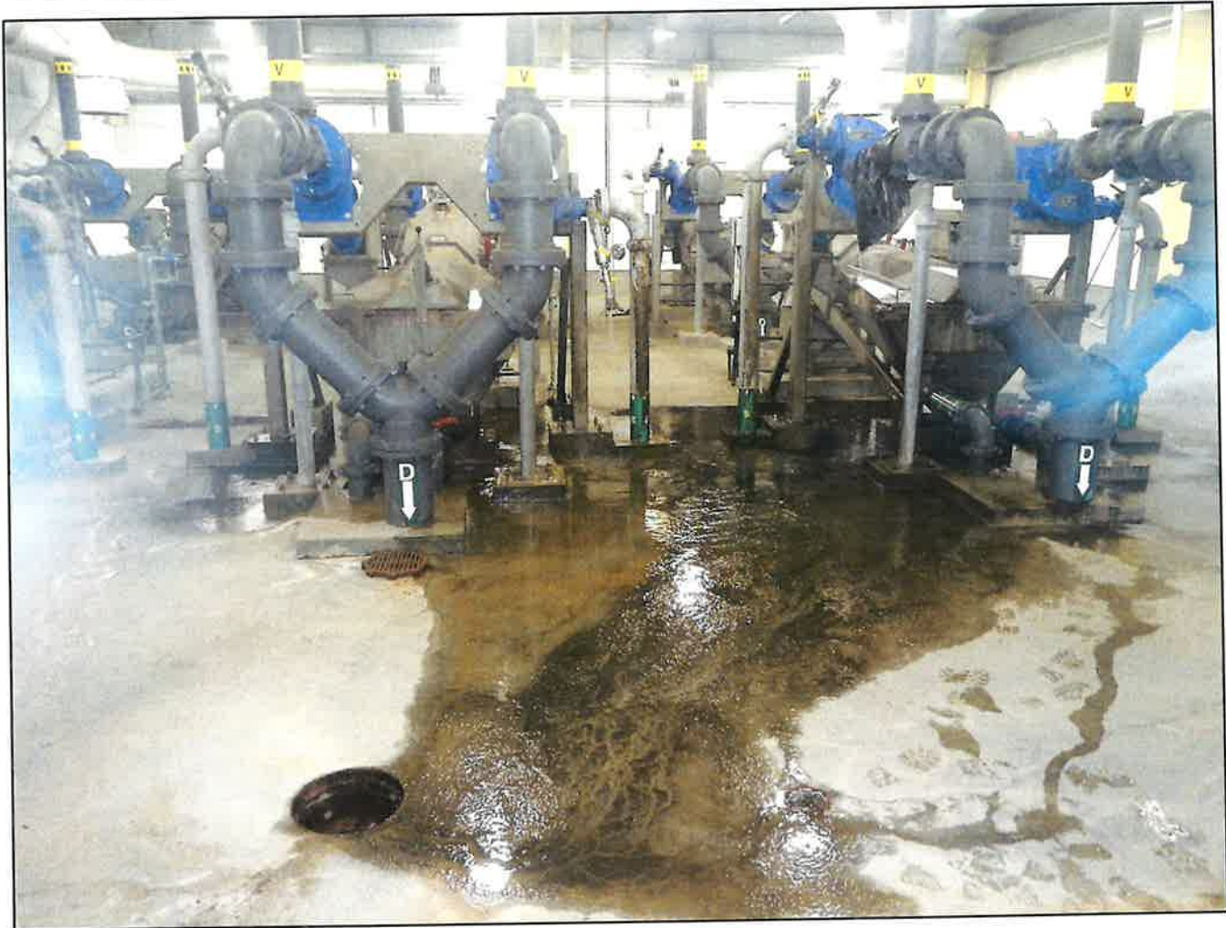
Photo 1. Primary Screening - Leaks from equipment seals on second floor of Grit Management Building; pictured are vortex separator Unit #1, classifier cell #1 and Unit 2, classifier cell #4.
