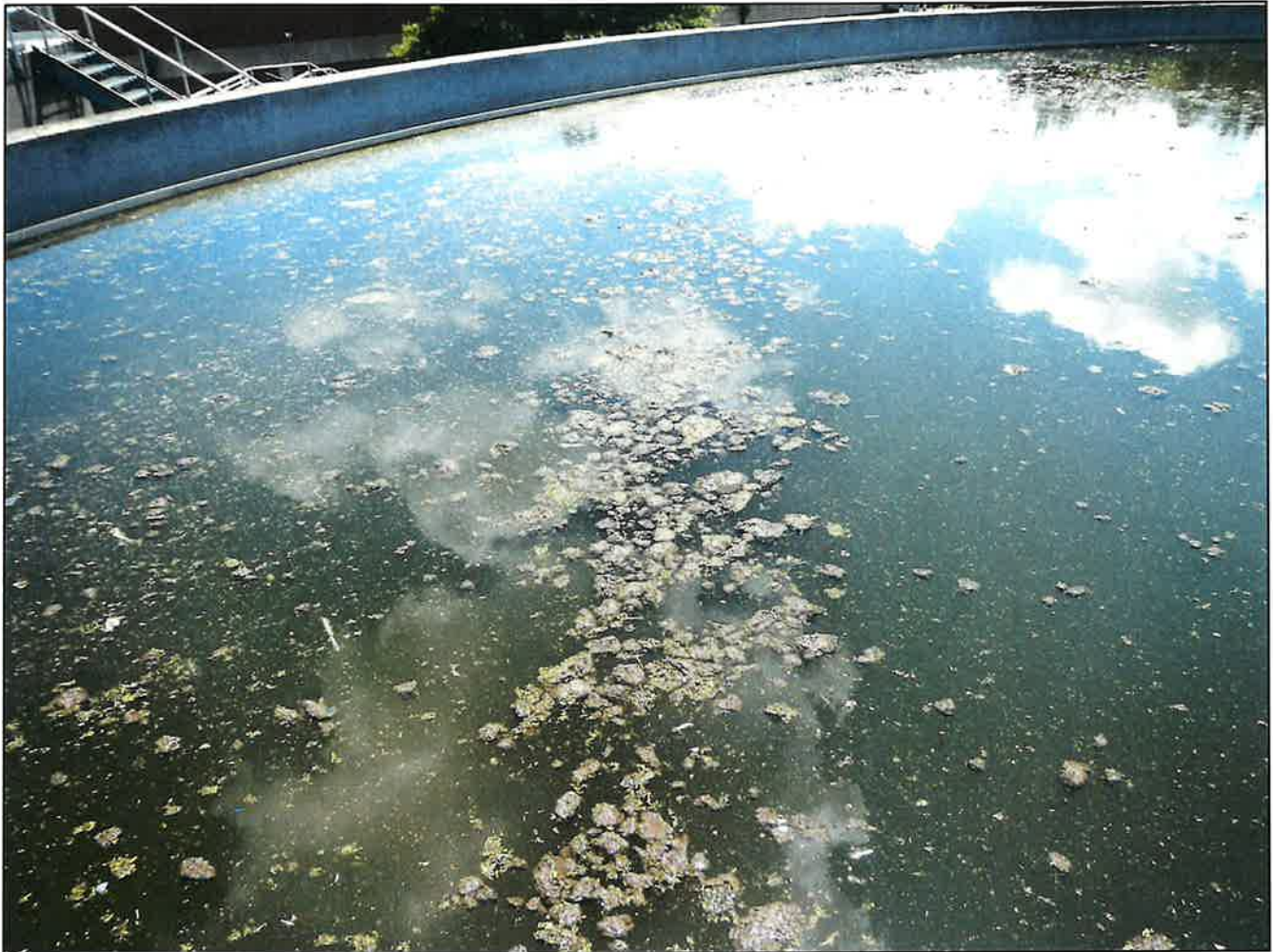
Photo 14. Secondary Clarification – Clarifier #6 with abundant floating solids.
