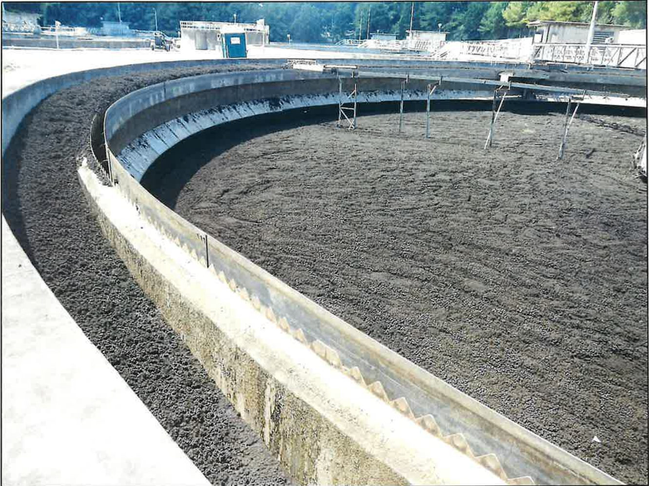
Photo 12. Secondary Clarification – Clarifier #5 (out of service) drained with evidence of solids blanket floatation that had extended beyond the outer weir into the effluent channel.
