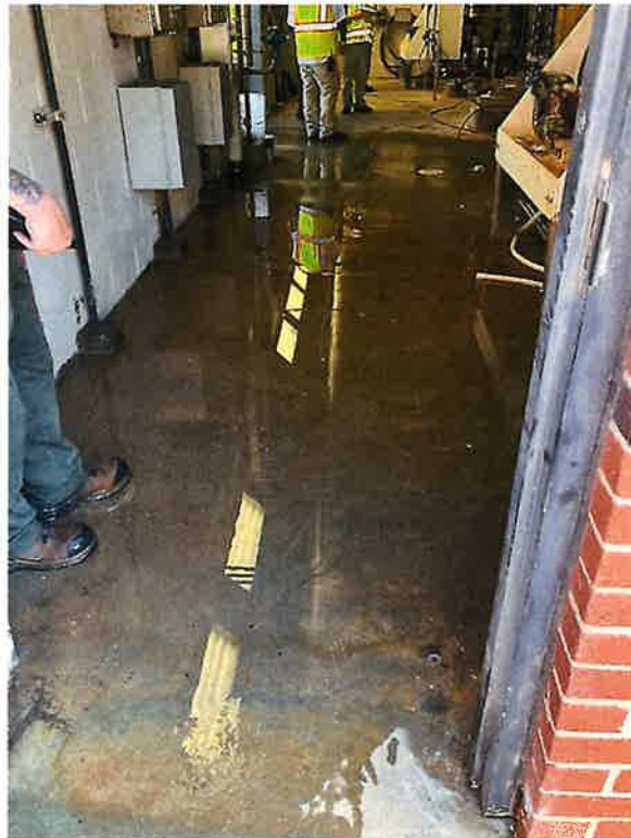
Photo 12: Water from Eyewash/Shower in Old Chemical Building
