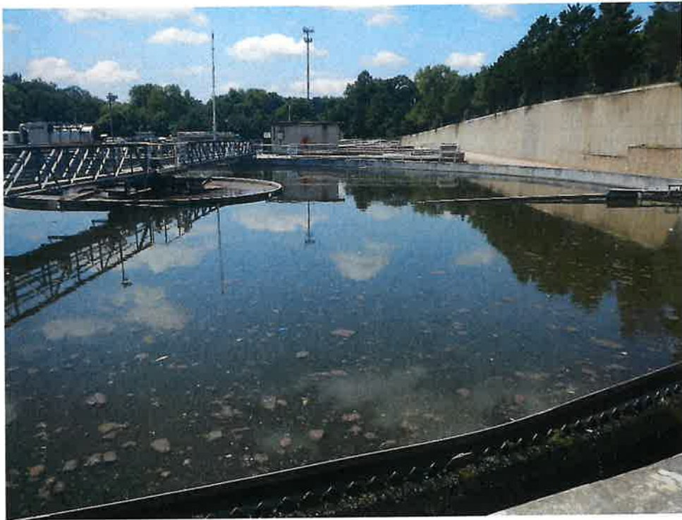
Photo 24: Secondary Clarifier #7 (picture provided by EPA)
