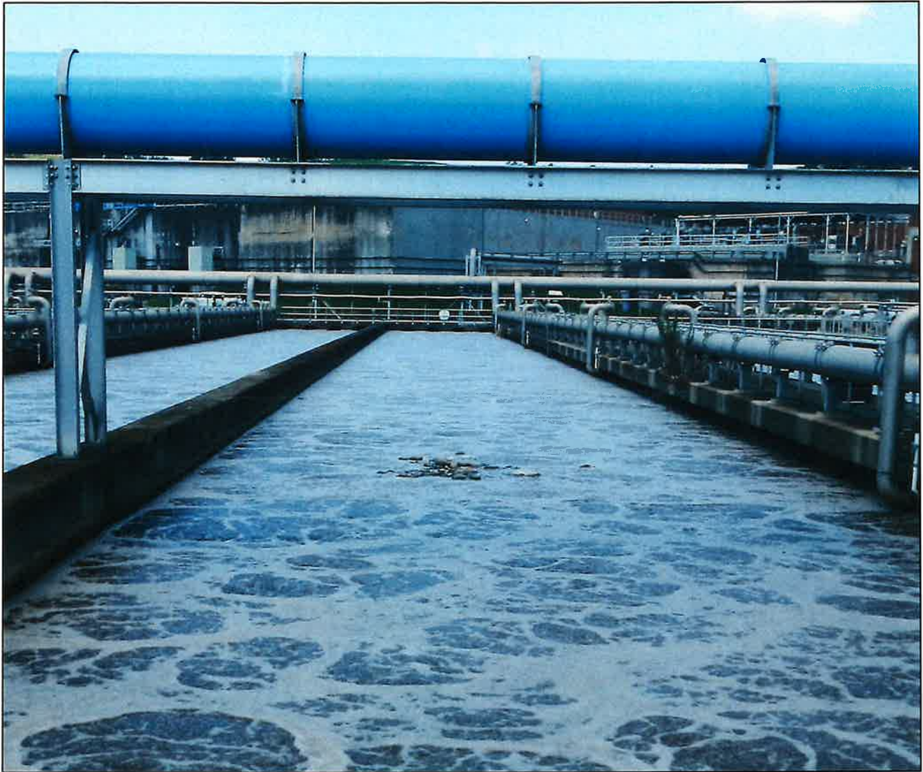
Photo 9. Biological Nutrient Removal (“BNR”) – Floating unscreened solids in BNR Tank #13.
