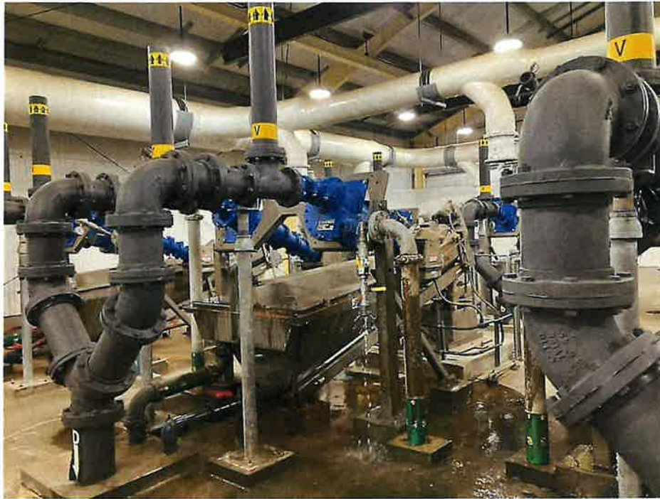
Photo 5: Damaged Grit Classifier (1)
