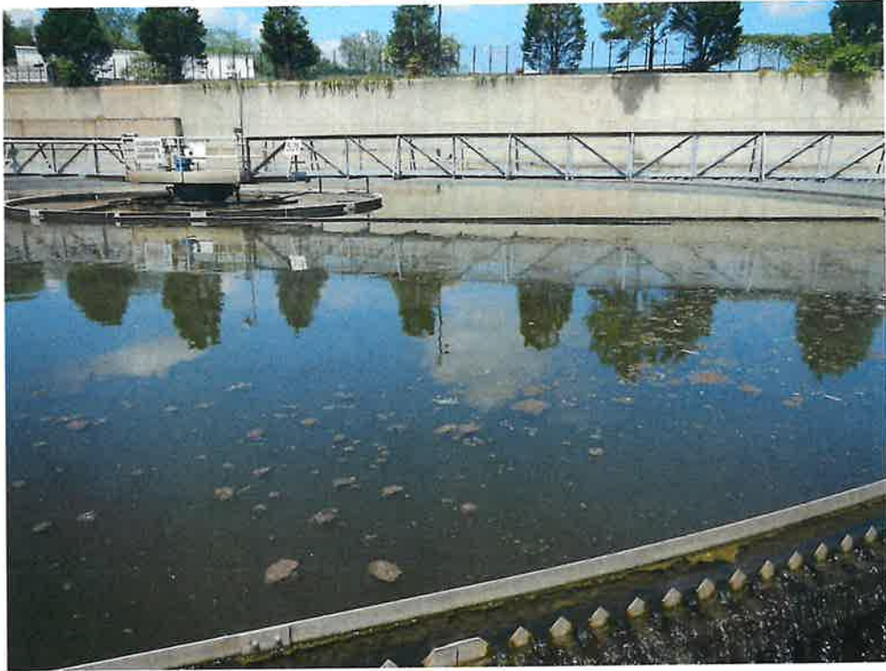
Photo 23: Secondary Clarifier #9 (picture provided by EPA)
