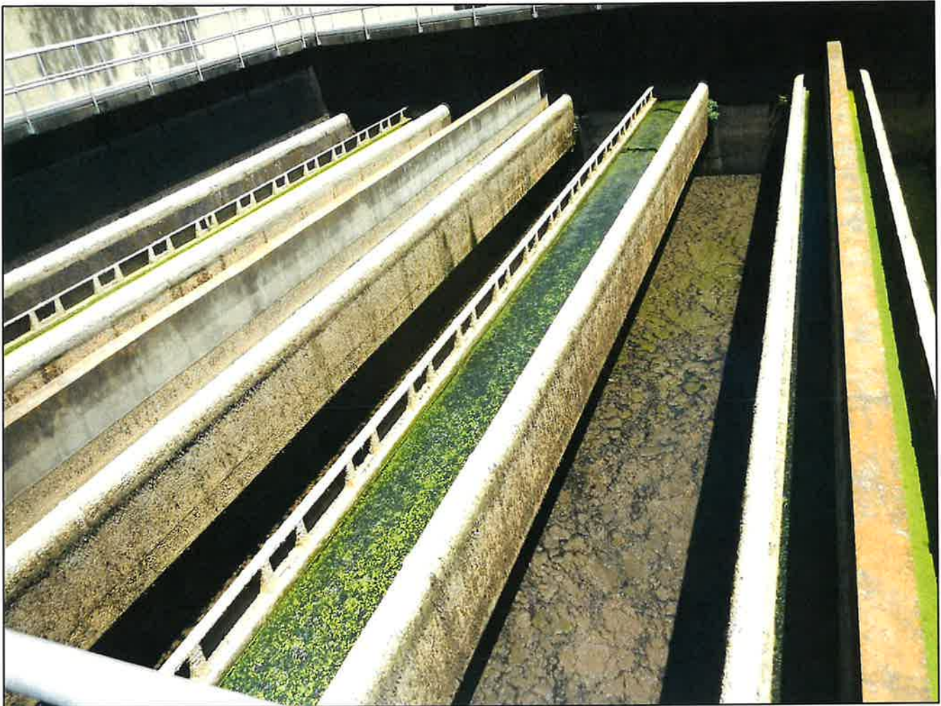
Photo 19. Tertiary Treatment – Media filters #18, 20, and 22 (out of service).
