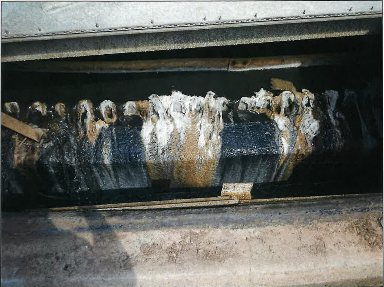
Photo 6. Primary Clarification – Debris and algal buildup on weirs, and evidence of solids passage over weirs; pictured is primary clarifier #4.
