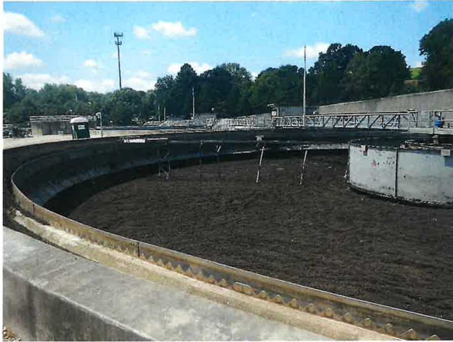
Photo 25: Secondary Clarifier #5 (picture provided by EPA)
