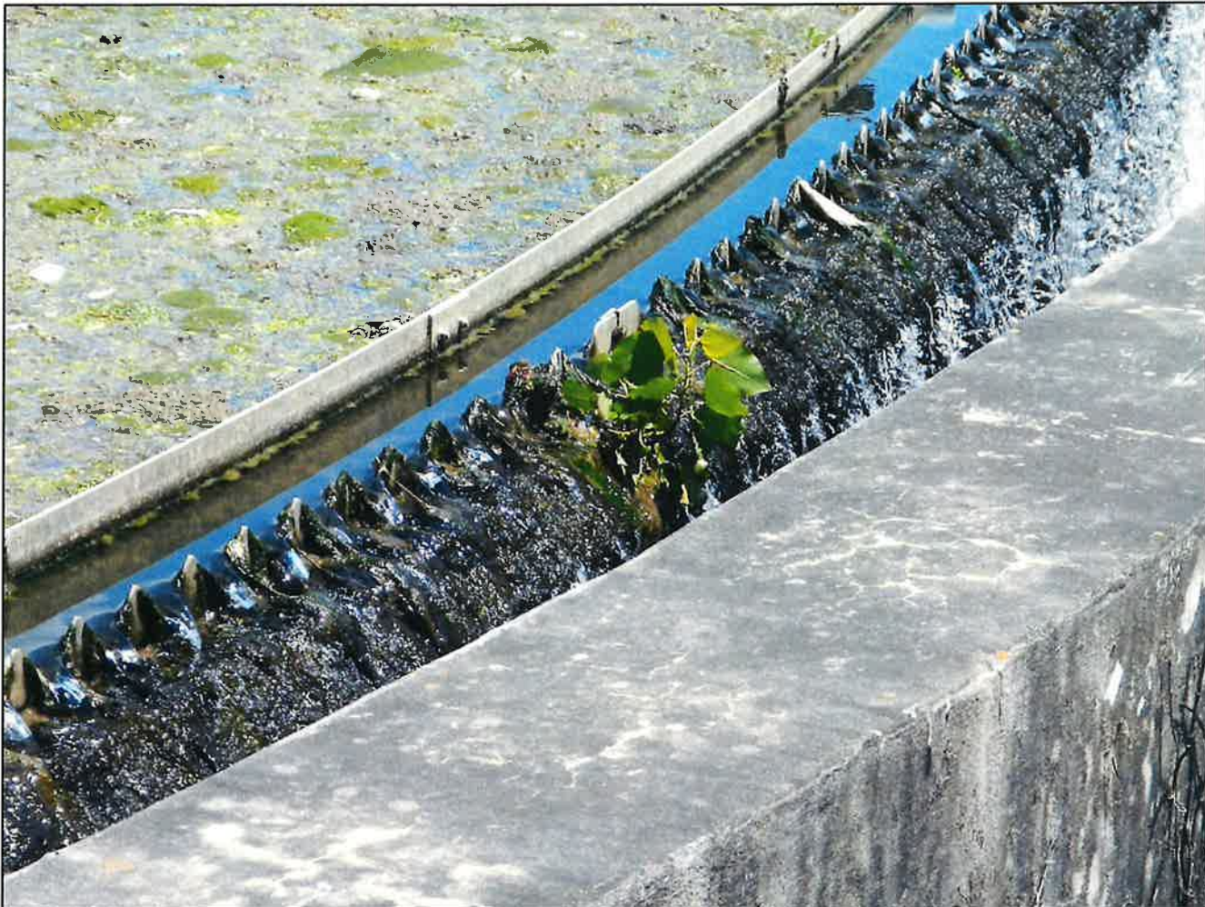
Photo 11. Secondary Clarification – Clarifier #10 with advanced plant growing out of effluent weir among abundant algal growth and debris depth built up on the weir and effluent channel.
