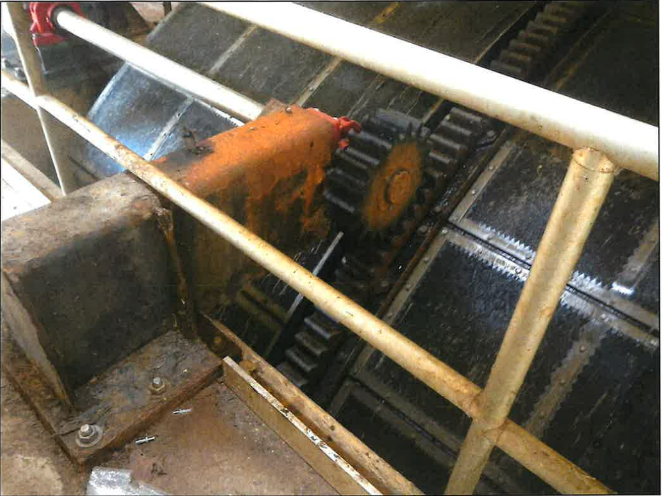
Photo 3. Primary Screening – Rusted drive cover of fine mesh screen drum #2 in Drum Screen Building.
