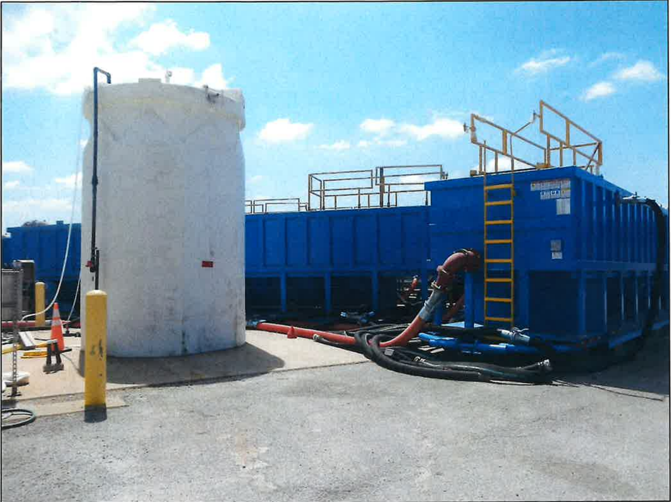
Photo 10. Temporary sodium hypochlorite tank and mobile secondary clarifiers installed between the Facility's secondary clarifiers and tertiary treatment.
