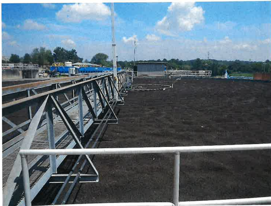
Photo 28: Secondary Clarifier #8 (picture provided by EPA)
