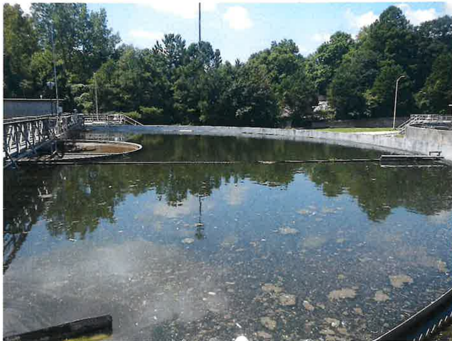
Photo 26: Secondary Clarifier #2 (picture provided by EPA)
